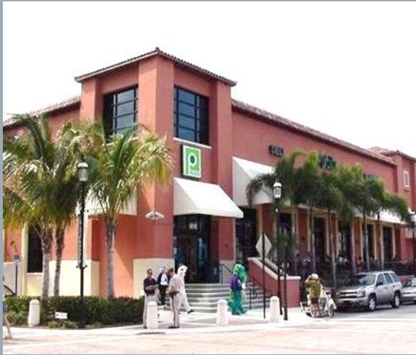
Steps extending into Street Setback Zone
